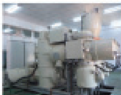
66/11 KV, 2 X 30 MVA GIS SUBSTATION @ YADANA
