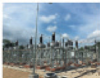
66/11 KV, 5 MVA SUBSTATION @ VERTICAL WIND TUNNEL
